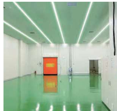
Ceiling panel with built-in LED lights
